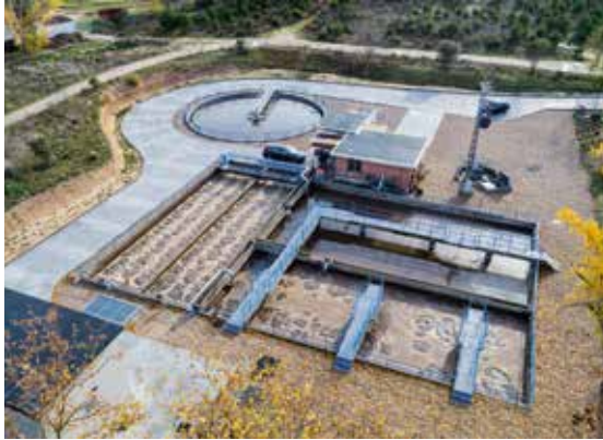
Wastewater treatment plant serving the Autonomous Uni- versity of Madrid (UAM) / Spain
